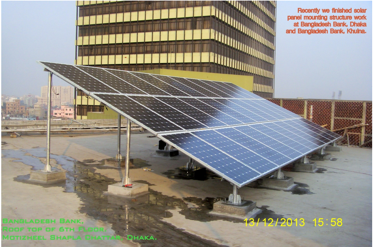
Solar Panel Mounting Frame Structure project at Bangladesh Bank, Motizheel Shapla Chattar, Dhaka. (15 kw )
