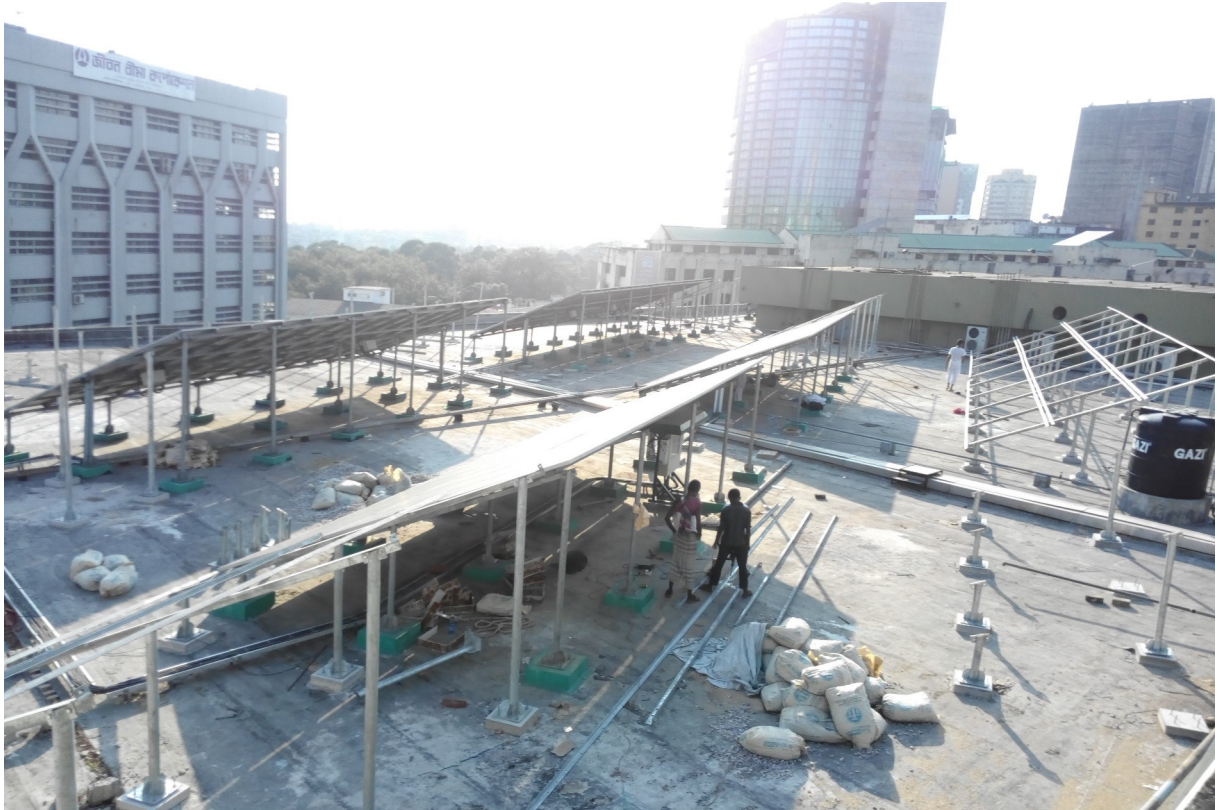
Solar Panel Mounting Frame Structure project at Bangladesh Bank, Shapla Chattar, Motizheel, Dhaka. (100 kw)
