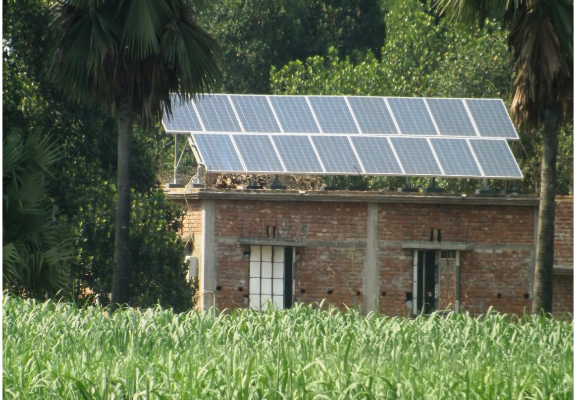
5KW Solar Power pump with Mounting Frame Structure project for PUMP-2 at Giashpur Bazar, Kapashia, Gazipur.
