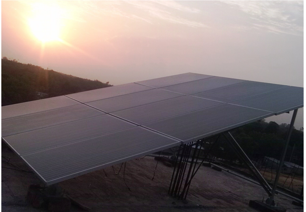
3KW NANO GRID Solar Power plant with Mounting Frame Structure project for K-3 at Amraid Bazar, Kapashia, Gazipur.
