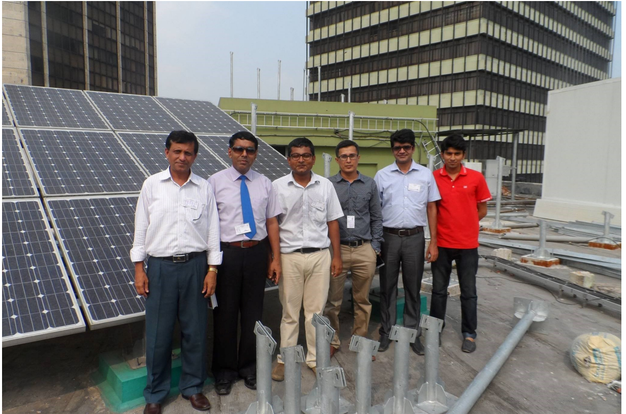
Solar Panel Mounting Frame Structure project at Bangladesh Bank, Shapla Chattar, Motizheel, Dhaka. (100 kw)
